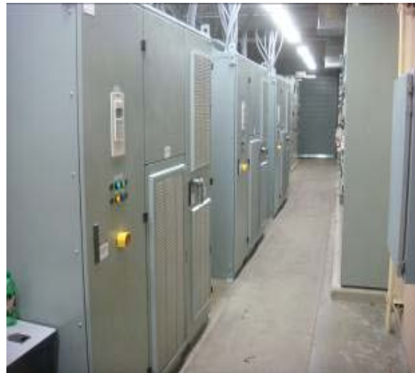
Three of the Six New ABB Medium Voltage VFDs
