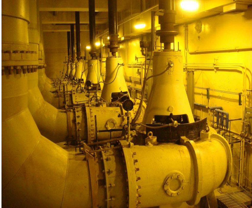
View of the Pump Gallery
